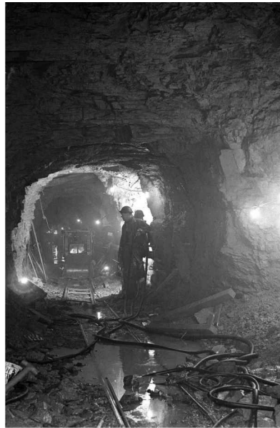
Working in the low active effluent tunnel, 46m below sea level. It's always night down here during the three-shift 24 hour working day. Taken in 1956/57.
