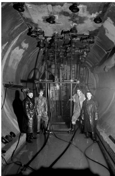
We're all very happy now, if not a little wet. Pipes 1-4 are now drilled above the 6" mild steel pipes and are now connected to the discharge system. Late 1957.
