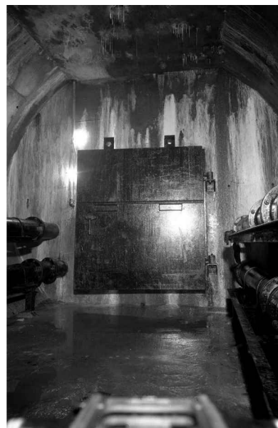
The view from inside the old diffuser chamber at the bulkhead door. Two 9" effluent pipes can be seen on either side of the chamber. The chamber is at the top of a 1:200 incline towards the base of the shaft. Late 1957.
