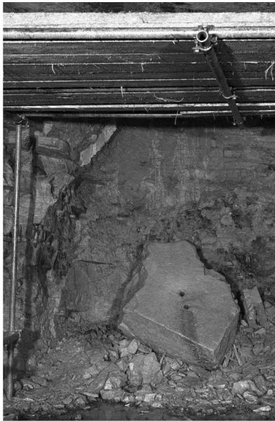
Scaffolding in the old diffuser chamber during construction. The layers of Caithness flagstone can be clearly seen on the left hand side of the photo along with the drill holes used to blast the rock during tunnel excavation. September 1957.
