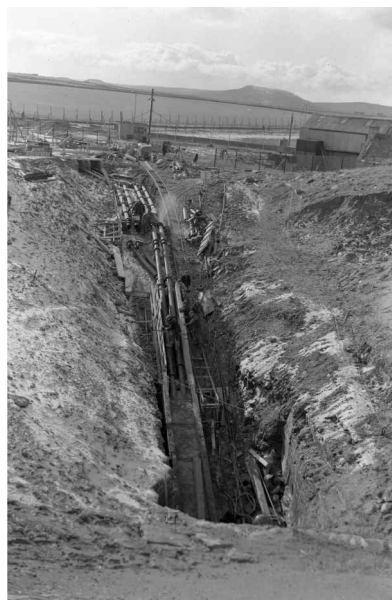
Securing the four 9" diameter cast iron effluent pipes into the adit by encasing in concrete haunching. The pipes lead up to the D1211 sea discharge pits. Taken in late 1957.
