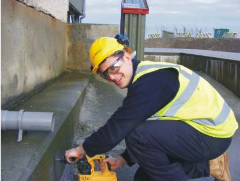
JCL mechanical technician Jason Orton extends the downpipe drain at the shaft.
