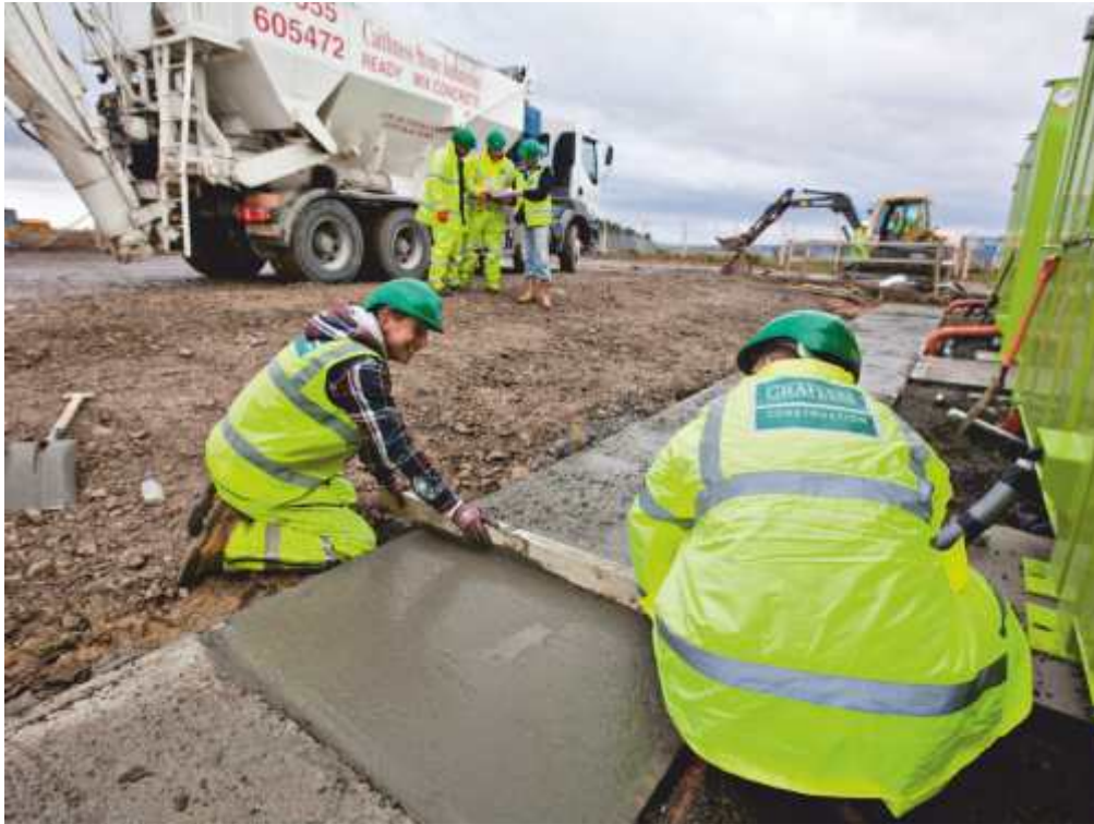
GRAHAM workers prepare the ground for the start of excavations later this month.
