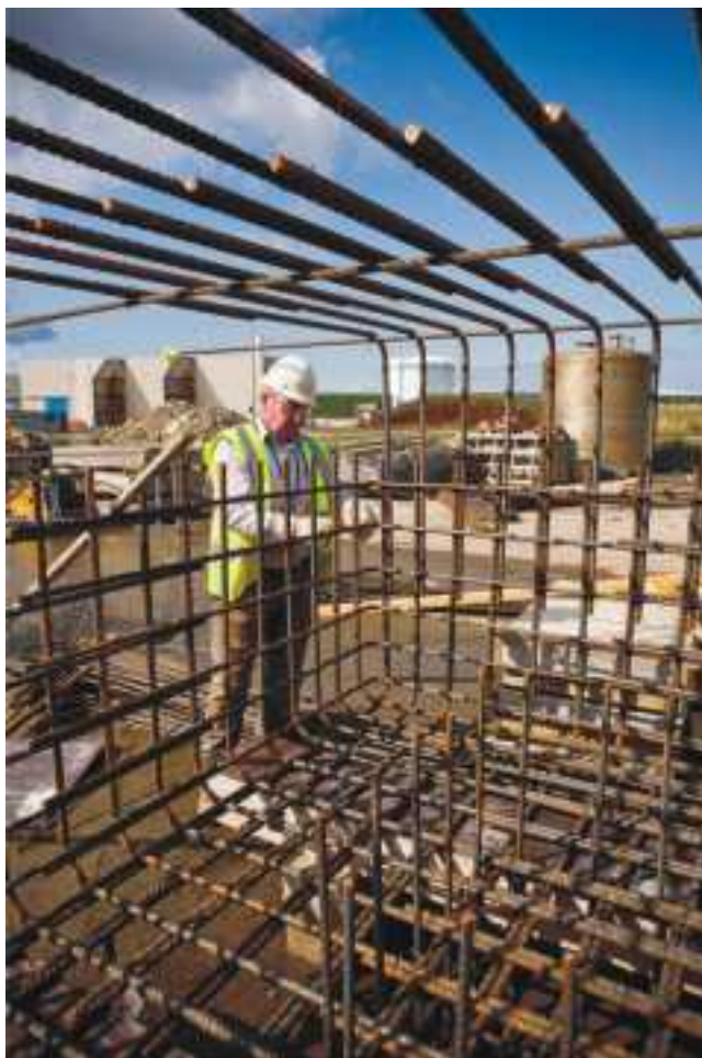
Derry Ross , foreman/steel fixer (Budge Formwork) working on the rebar for the stack foundation. The stack will sit on top of 59 tons of reinforcement bar and concrete.
