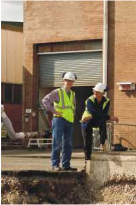
Project manager Iain Lyall (DSRL) and project supervisor Jim Mackenzie (DSRL) checking the foundations for the stack.
