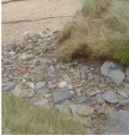
Figure B-1: Storm damage to Sandside path
