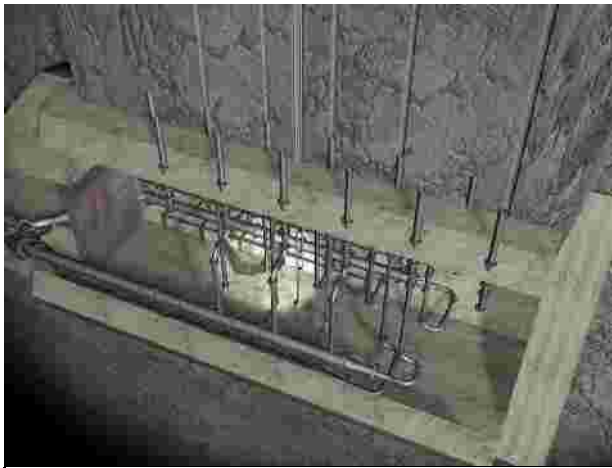
Diffuser Chamber – Constructed in 1956, 23m below seabed, 600m from shore at the end of the effluent tunnel.
