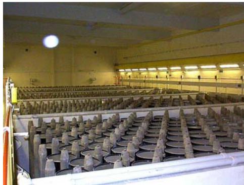
Figure 28: View inside CHILW drum store
