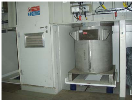
Figure 23: DFR Ion Exchange Column inside transport overpack
